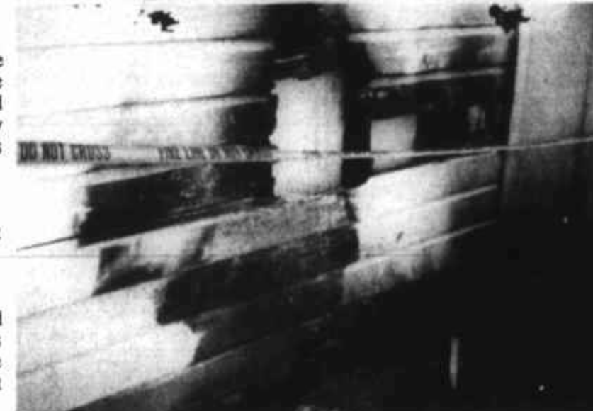
Arson is suspected in the fire which burned holes through the back wall of JJ's Chicken located on W. Main in Eagle Lake. Quick action on the part of the Eagle Lake Police Department and Volunteer Fire Department saved the building from further damage.
